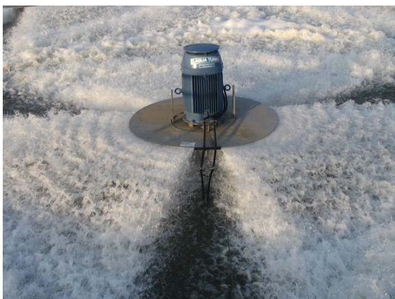
Discharge is directed away from the motor.
