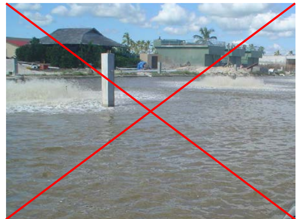
Small oxygen dispersion – 18.5kW = 20mØ. Pump action is lost from basin by throwing water vertically.
