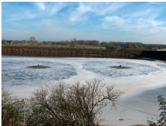
Large oxygen dispersion – 18.kW = 90mØ. Pump action translates to horizontal mixing energy in basin.
